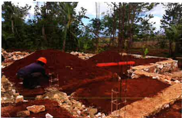
ABOVE : Construction on a new home being built in Musotte after the hurricane.
